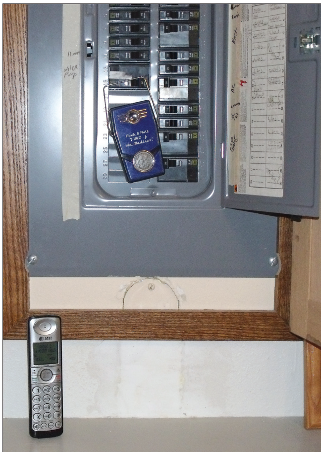
Figure 1 — AM receiver shown hung on a switch of the circuit breaker panel, with the telephone/intercom below. [Michael Foerster, WØIH, photo]
