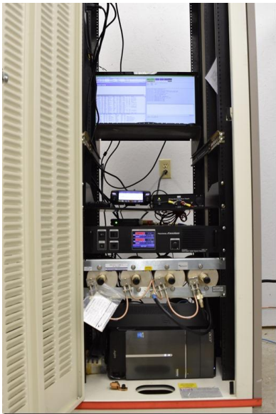
Figure 2 UHF CALDWELL CO REPEATER
